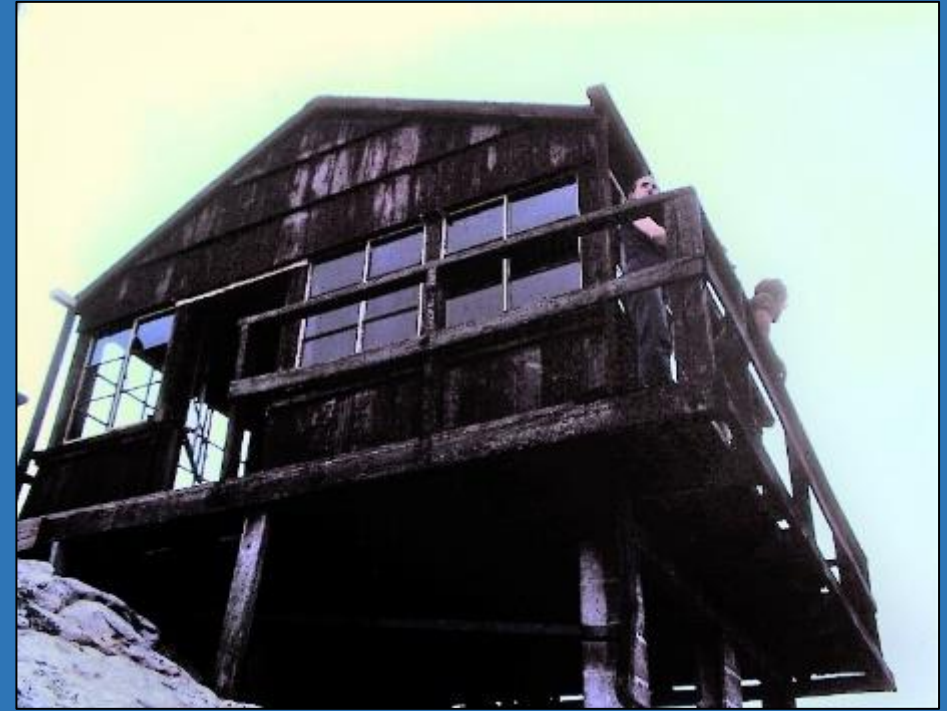
This 1980 image of the old fire observatory shows broken window panes, weathered wood, no door, and no stairs. (Doug Wood photo).
